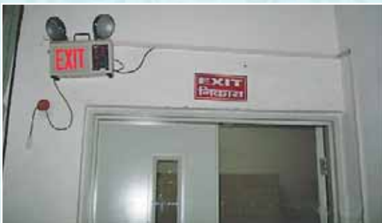
Emergency Light/ Exit Opening Outwards
